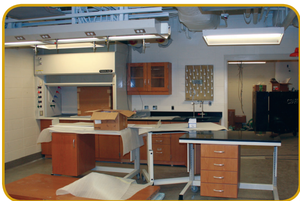
This open-concept research lab is part of Phase I of the renovation, and used to be rooms G5, G7 and G9.
